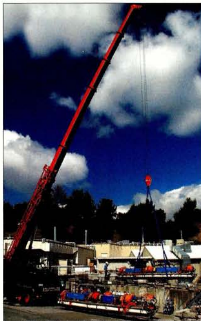
A crane removes the "rafts" of SPEAR2 on 22 April this year, in preparation for the construction of SPEAR3.
